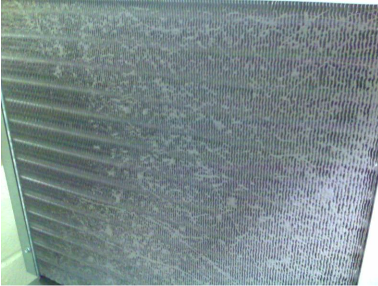
Condenser Coil in need of cleaning.
