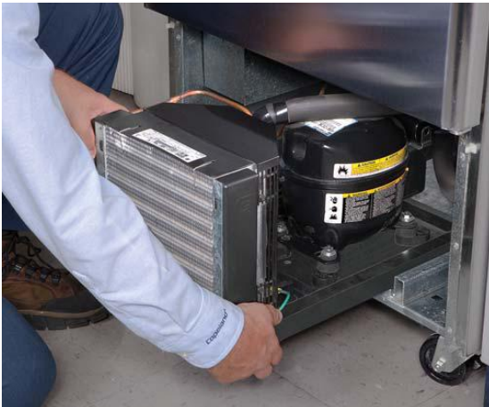
Clean Condenser Coil on a relatively new unit
