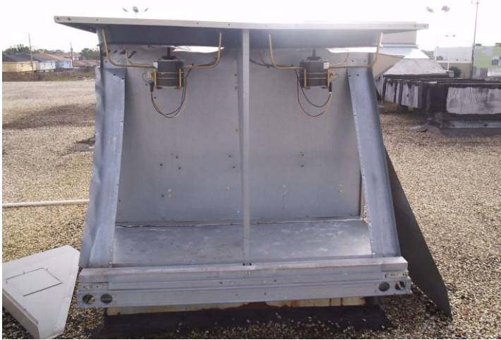
This relatively new unit was stripped by vandals for the scrap value of the copper coils. An excellent example of a reactive replacement candidate.
