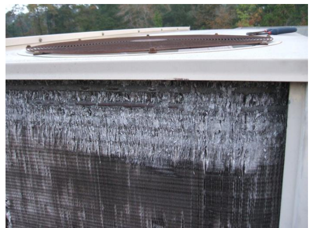
Corroded Condenser Coils Decrease Efficiency
