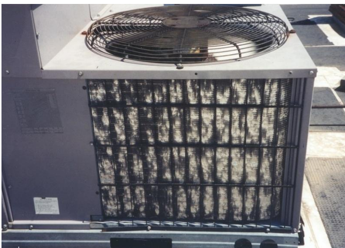
Hail Damaged Inefficient Condenser Coils
